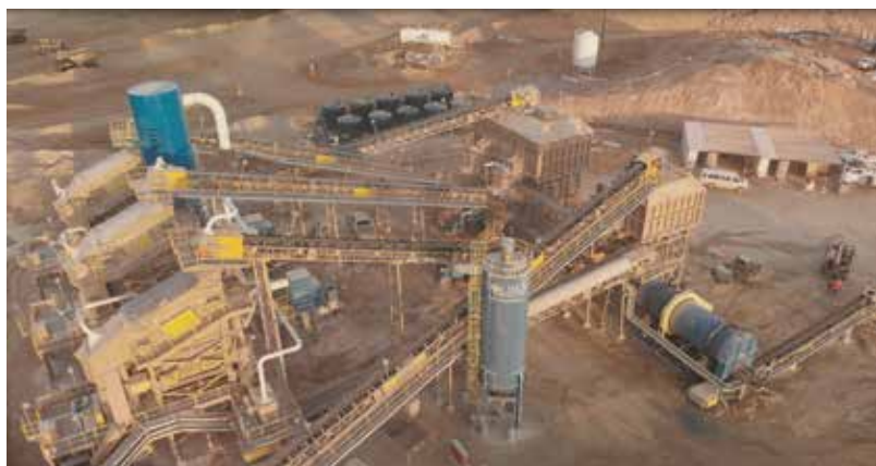
Crushers at the Moss gold/silver mine in northwest Arizona. Photo courtesy Northern Vertex Mining Corp.
